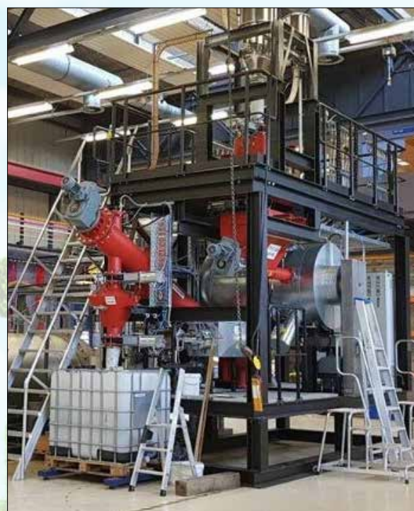
The results of the 1 MW pilot plant in Groningen led to the design contract for a 25 MW plant for Pörner.
