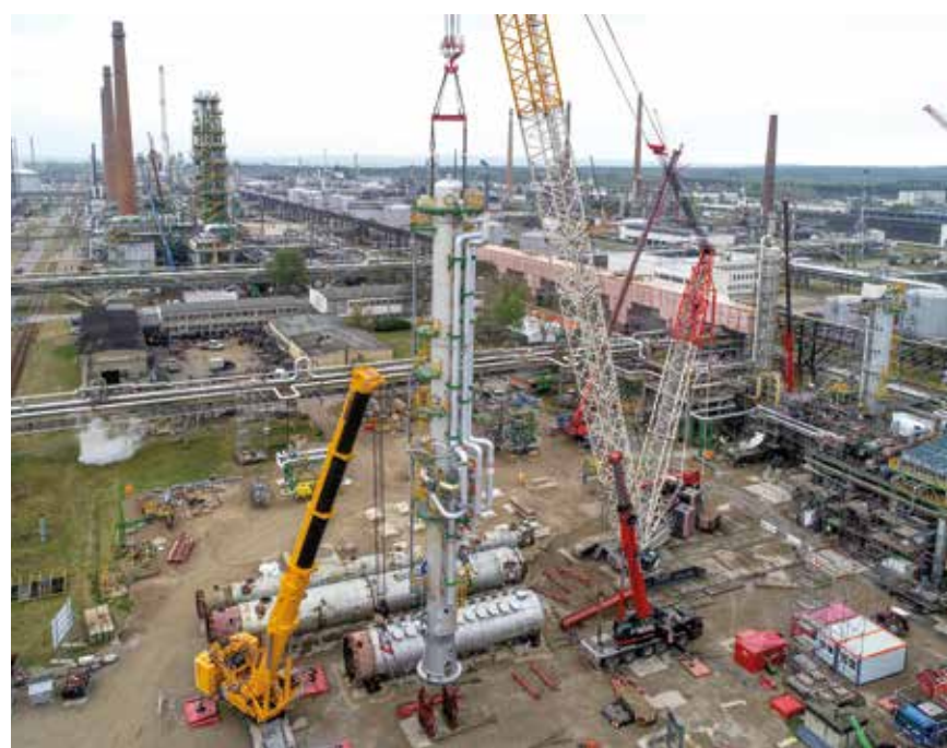
Aromatics extraction plant at the PCK refinery: Classic revamp with minimization of energy and operating material consumption combined with innovative EDL technology for extractive distillation to minimize of toxic solvents.
