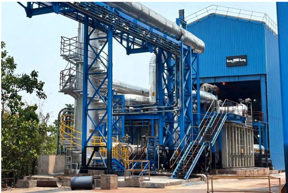
Fig. 7: The thermal energy storage system at Tata Steel's Sinter Plant 3.
